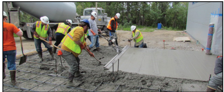
Peter Macchione, Jacob Pomeroy, Kelly Bowen, Heather Matumeak, Jeff Lucas, Mike Nolan and John Hudson pour concrete at the new training facility.
